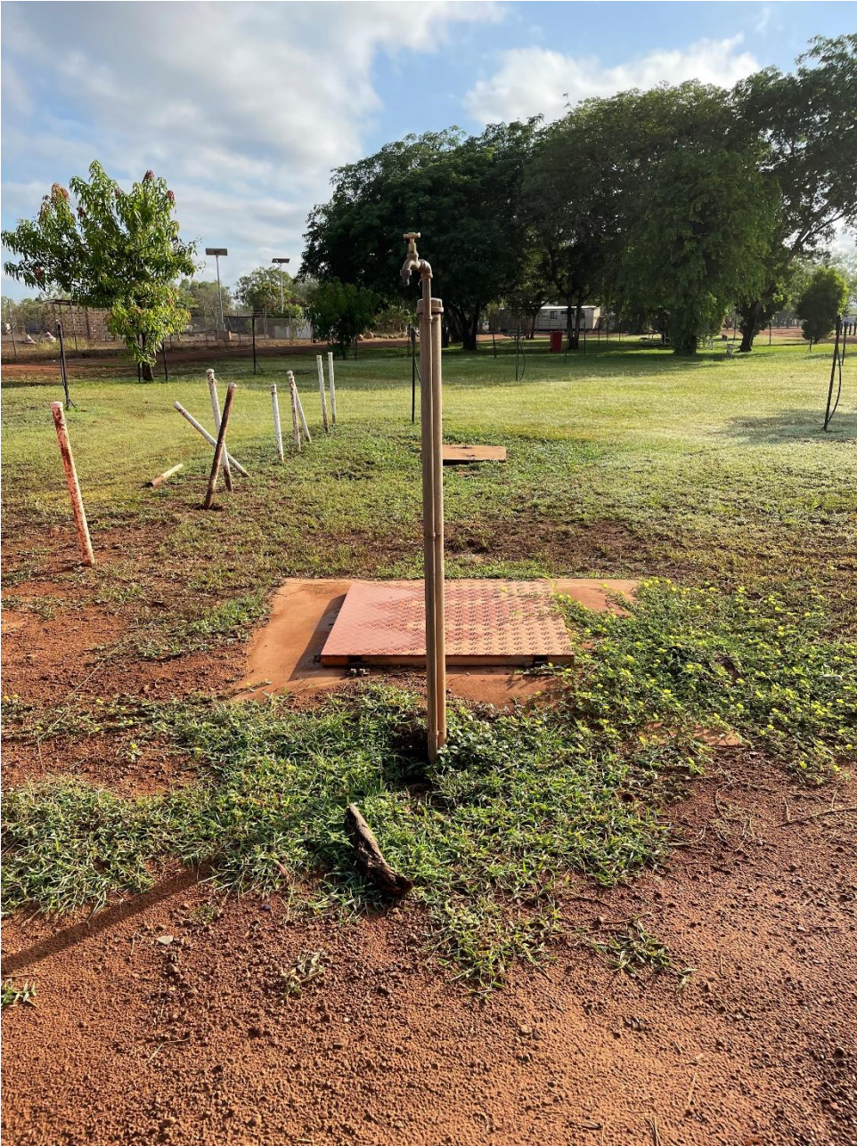
Figure 7: Existing sullage dump point showing the existing toilet block to the left in the background. This dump point is to be made redundant.
