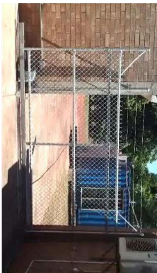
CHAINMESH SECURITY FENCING
