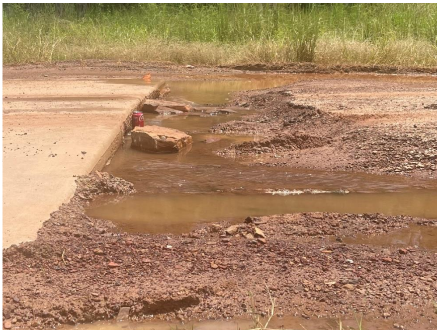
Image description: Road conditions at Garawa One town camp taken on Monday 13 March 2023 after minor flooding in Borroloola.
