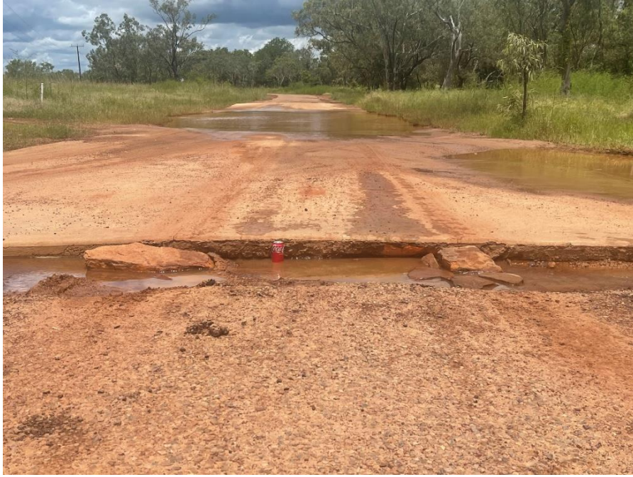
Image description: Road conditions at Garawa One town camp taken on Monday 13 March 2023 after minor flooding in Borroloola.
