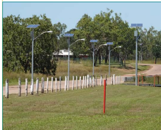
Solar lights at Beswick linking old and new subdivisions
